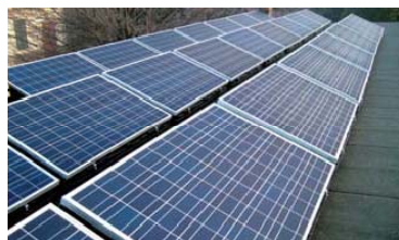
Figure 4.3: Solar PV Modules (Appendix 11.3 for Manufacturer's specifications of Solar PV Panels)
