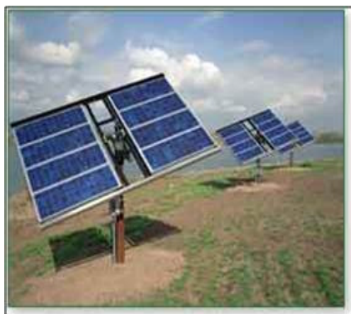
Figure 5 – 2: Solar PV pumping unit
