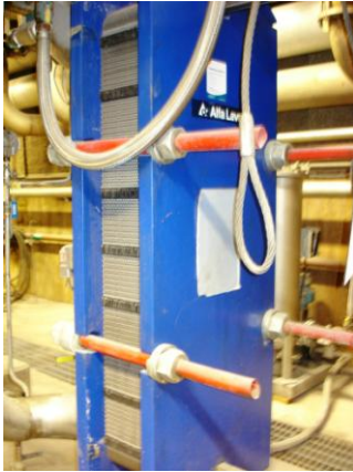
Figure 30 : KB2 Heat Exchanger
