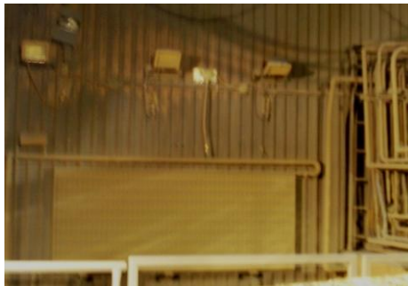
Figure 27: Cooling Water Radiators inside Cutting Line
